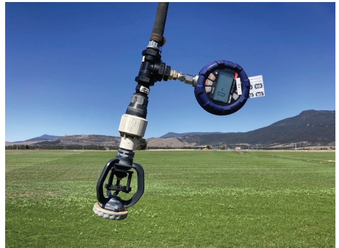
Pressure being measured above the regulator on the last drop tube
